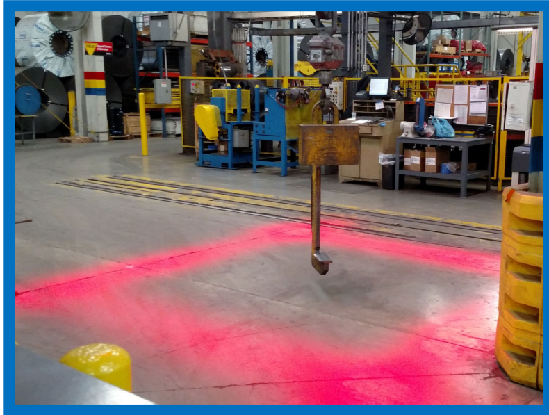
4 - Crane Lights with Lens - Quad Lines
